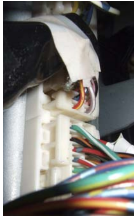
Plugs on AHC Unit
